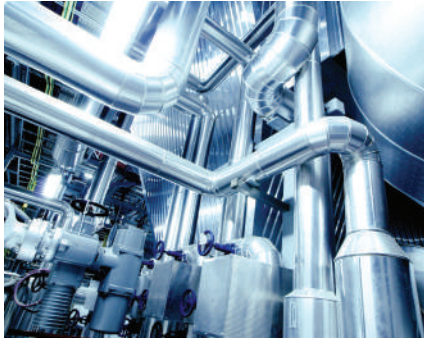
Typical high-corrosive environment — central utility plants.
