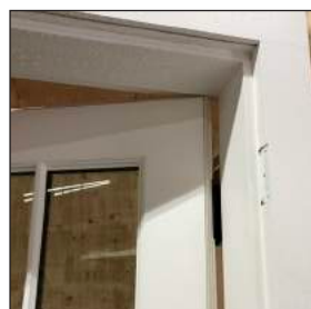
1/2" x 1/2" notched detail around the exterior door with two sets of 360° weatherstripping
